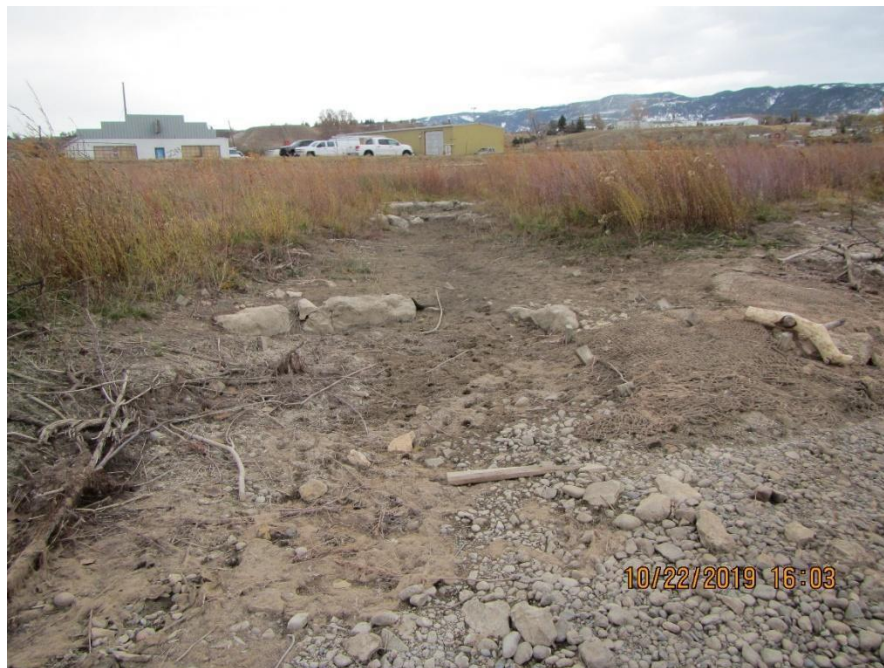
FIGURE A.5.22. Site 2 & 3 - Wyoming Blvd, at upstream set of wetland cross vanes, looking at cross vanes 39A (middle) and 39B (closest). Cross vane 38 is also visible (furthest).
