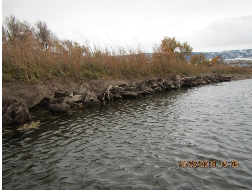
FIGURE A.5.5. Site 2 & 3 - Wyoming Blvd, at middle of toe wood 3 in-stream, looking at upstream half of toe wood 3.
