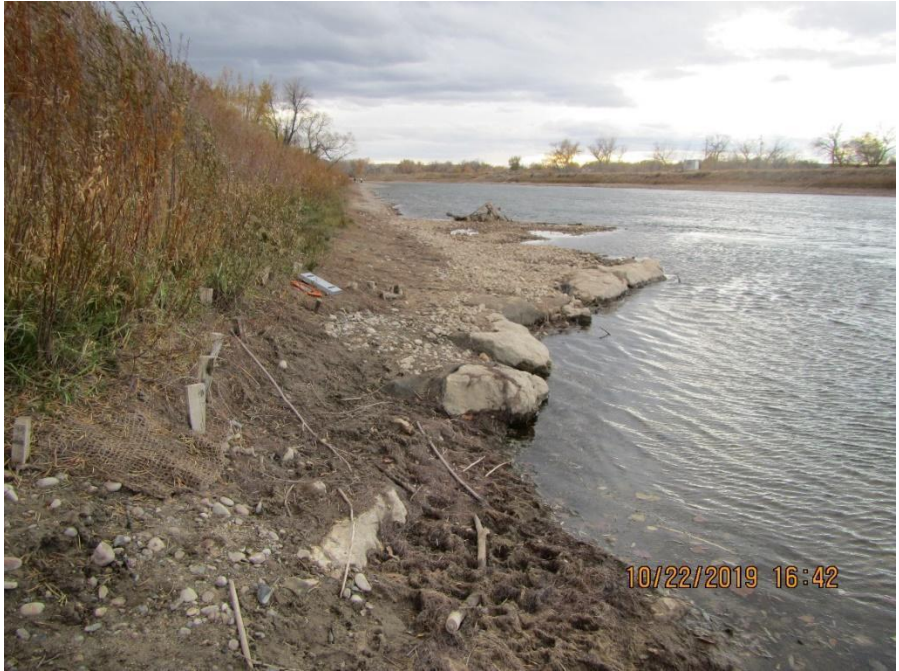
FIGURE A.5.11. Site 2 & 3 - Wyoming Blvd, standing downstream of rock vane 1 on river right, looking upstream.
